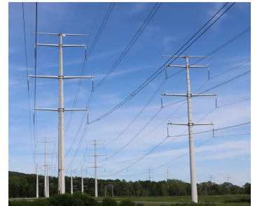
Figure 1.1 345,000 volt transmission lines.
